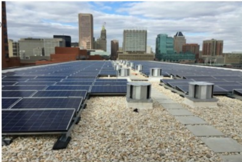
Sol's 196-kilowatt solar installation at Christ Church apartments, a low-to-moderate income senior living facility located on the Baltimore Harbor.
