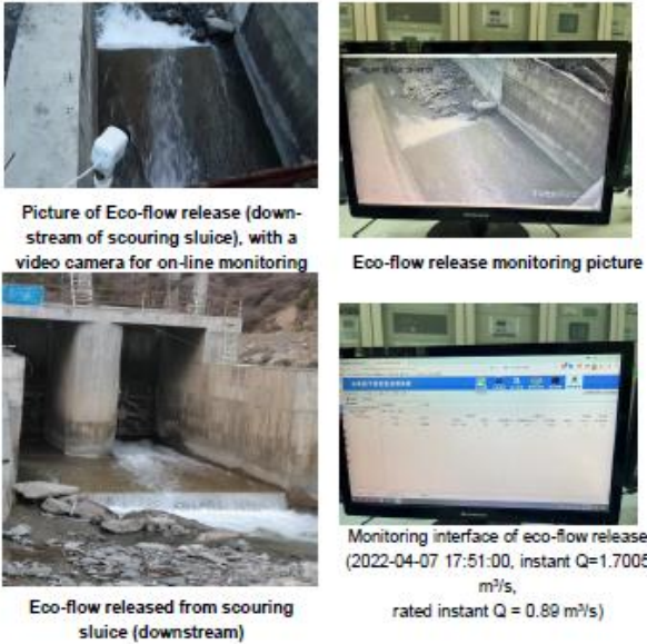
Figure 10 Site pictures on eco-flow release monitoring and operation
