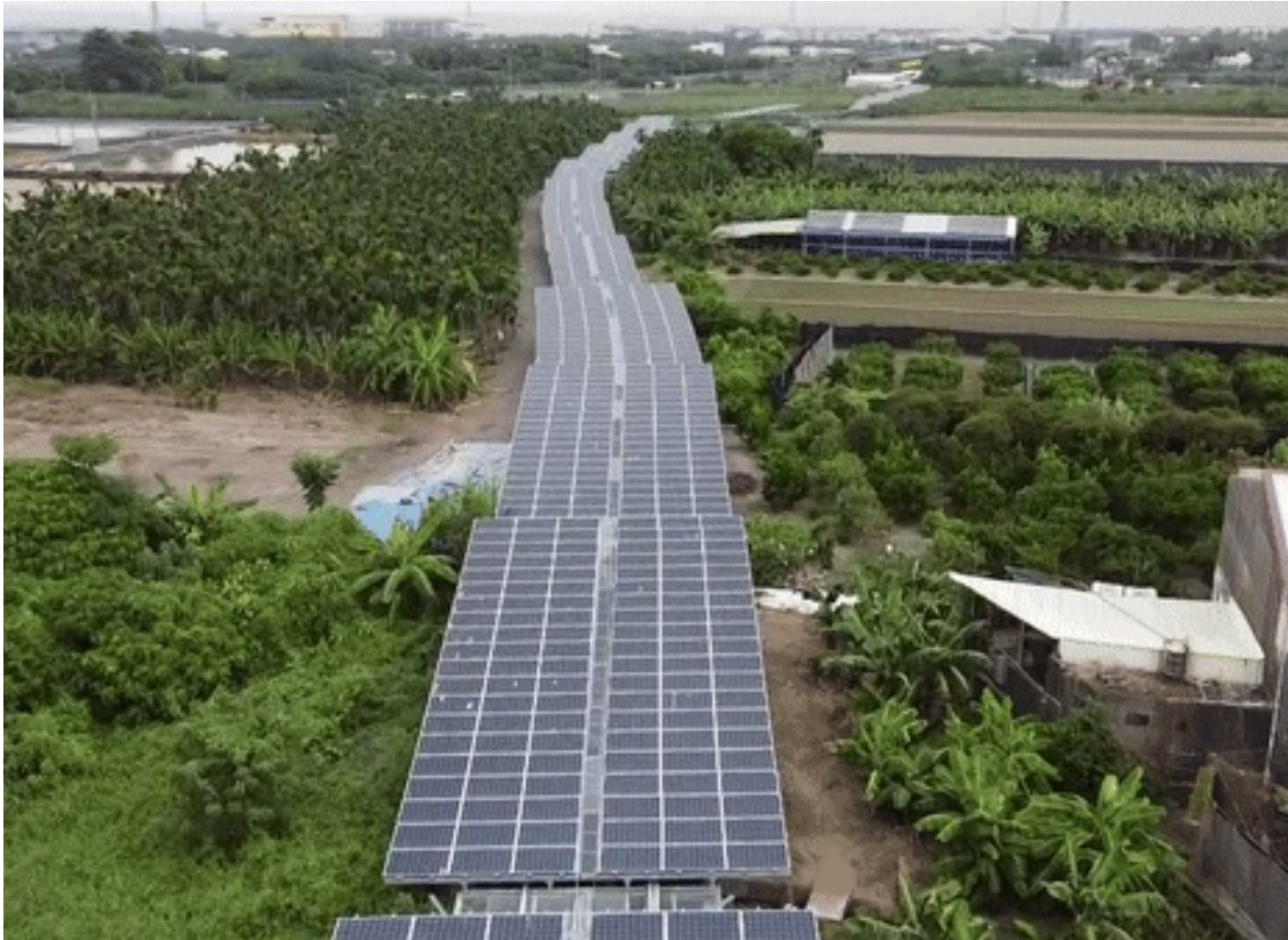
Pingtung Canal – 3.3MWp
