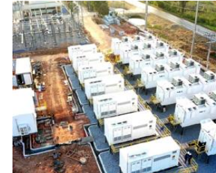
Chai Badan Substation
