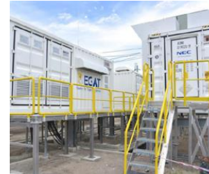
Bamnet Narong Substation
